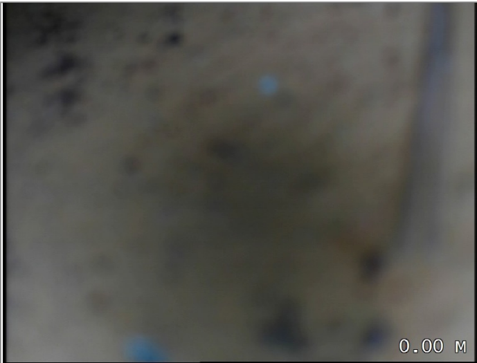
Start node type, manhole, reference MHF 4 LAT - A
