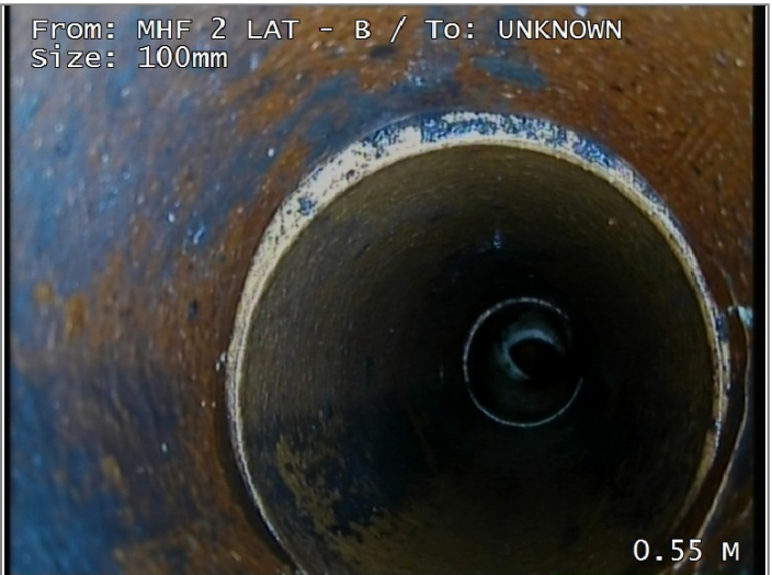
Cracks multiple from 12 to 12 o'clock
