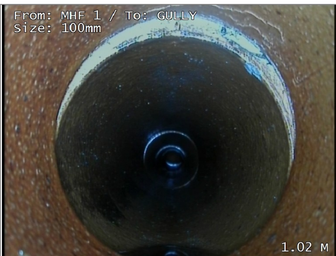
Crack circumferential from 12 to 12 o'clock
