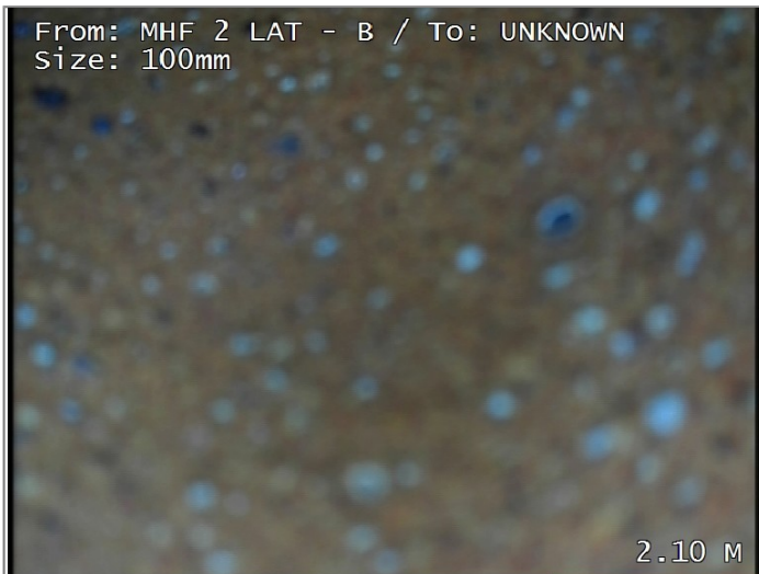
Line of drain/sewer deviates up
