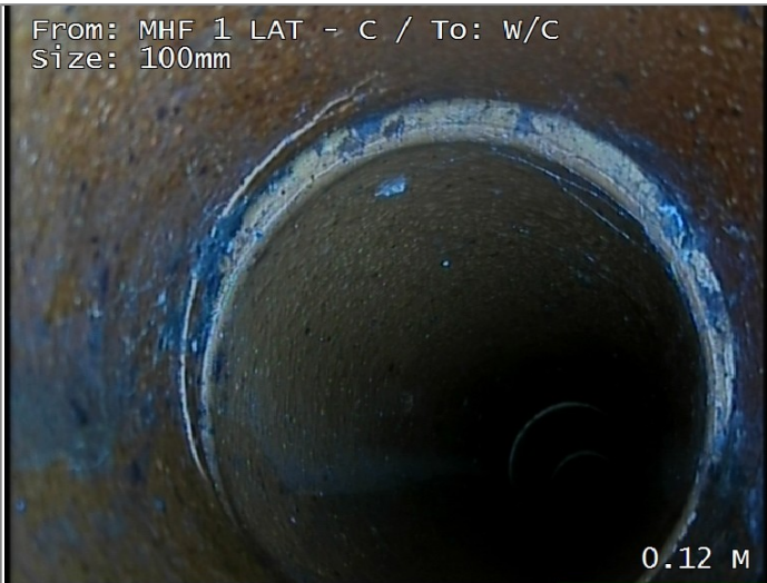
Crack circumferential from 12 to 12 o'clock
