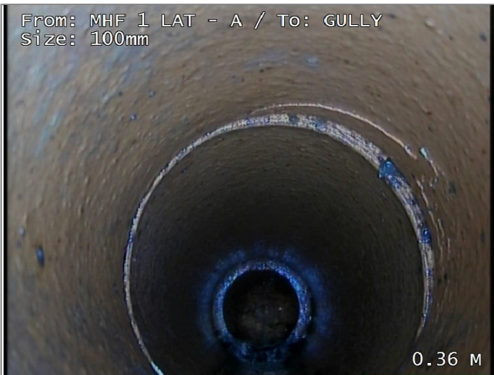
Crack circumferential from 12 to 12 o'clock
