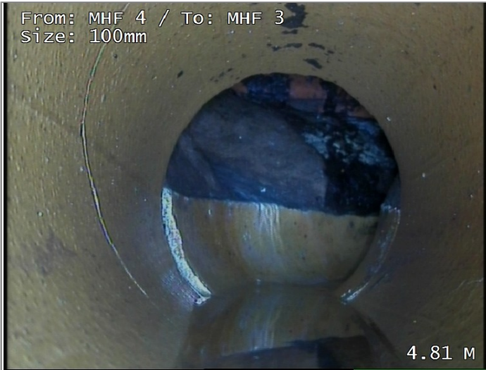
Crack circumferential from 12 to 12 o'clock
