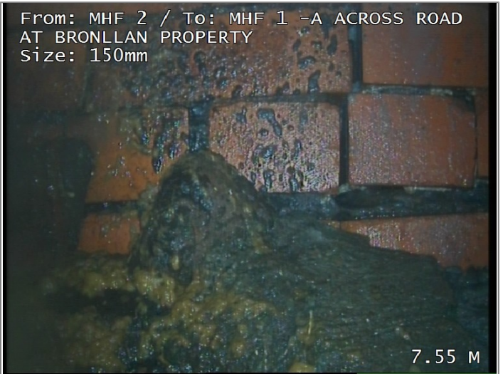
Finish node type, manhole, reference MHF 1 -A ACROSS ROAD AT BRONLLAN PROPERTY
