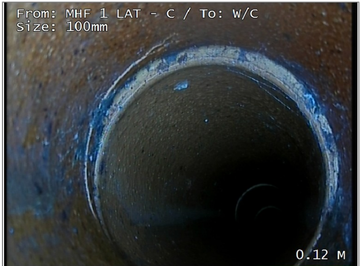
Line of drain/sewer deviates right
