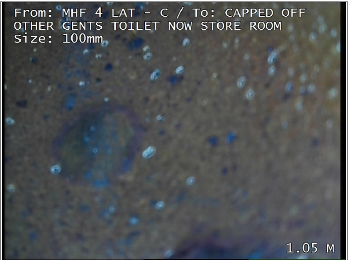
Line of drain/sewer deviates up
