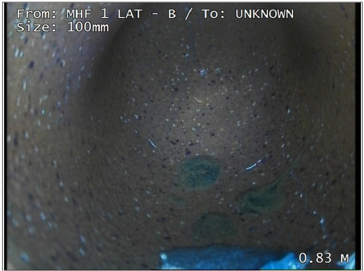
Line of drain/sewer deviates up
