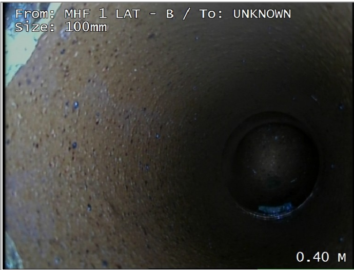
Line of drain/sewer deviates right
