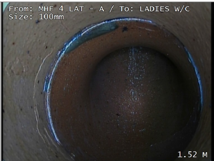
Crack circumferential from 6 to 12 o'clock
