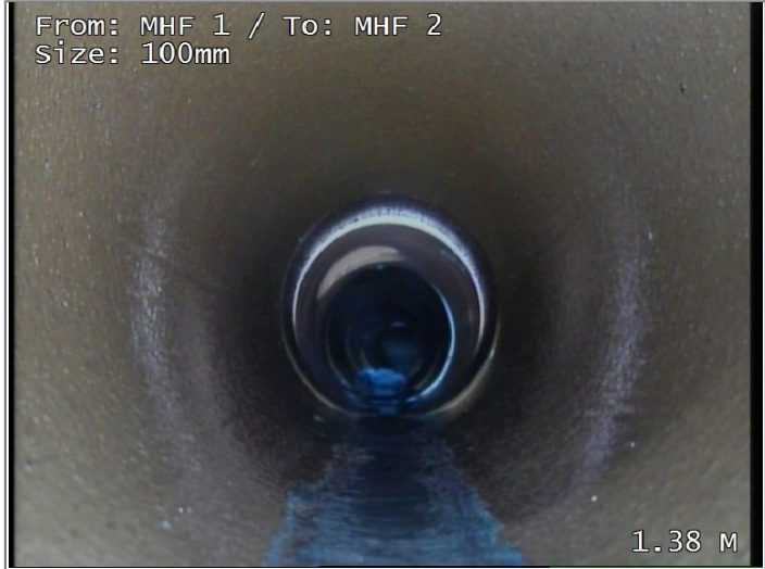
Length of individual pipe forming drain/sewer changes at this point, new length 150mm
