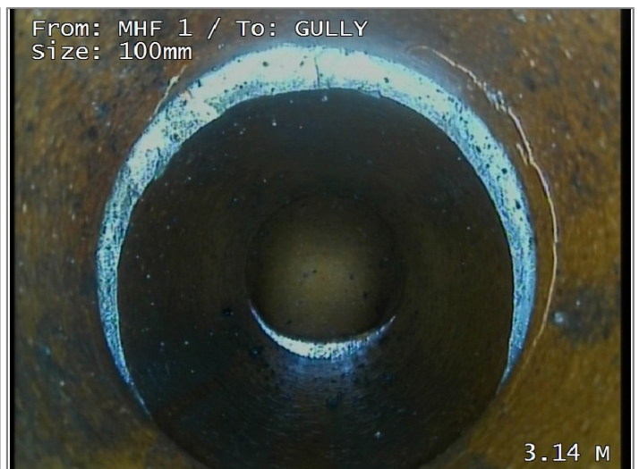
Joint displaced medium
