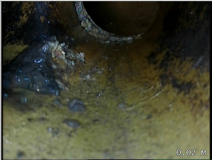
Start node type, manhole, reference MHF 4 LAT - C
