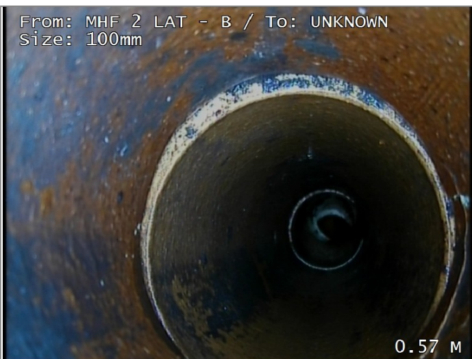
Joint displaced medium
