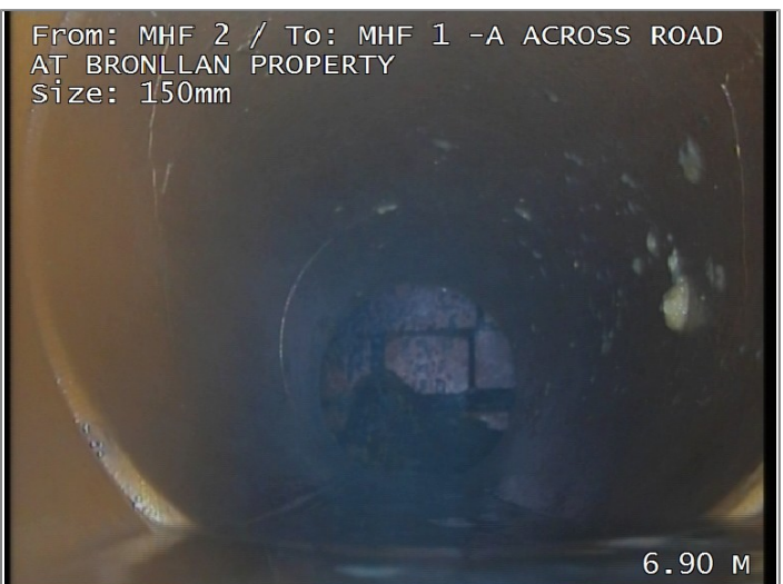
Cracks multiple from 12 to 12 o'clock
