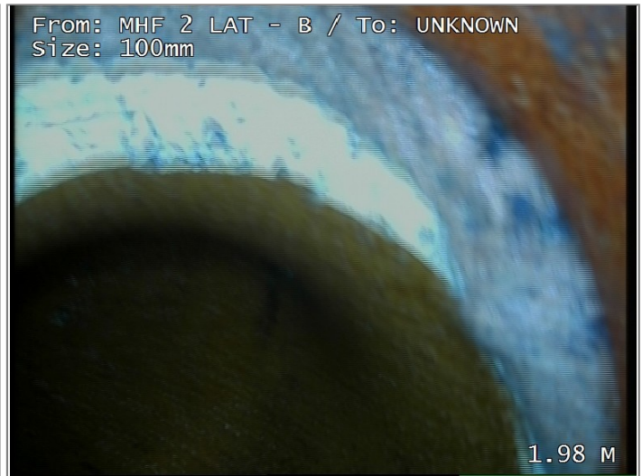
Joint displaced large
