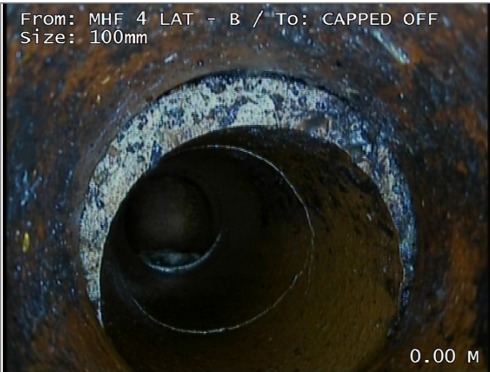
Joint displaced medium
