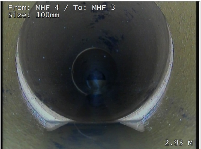
Joint displaced medium
