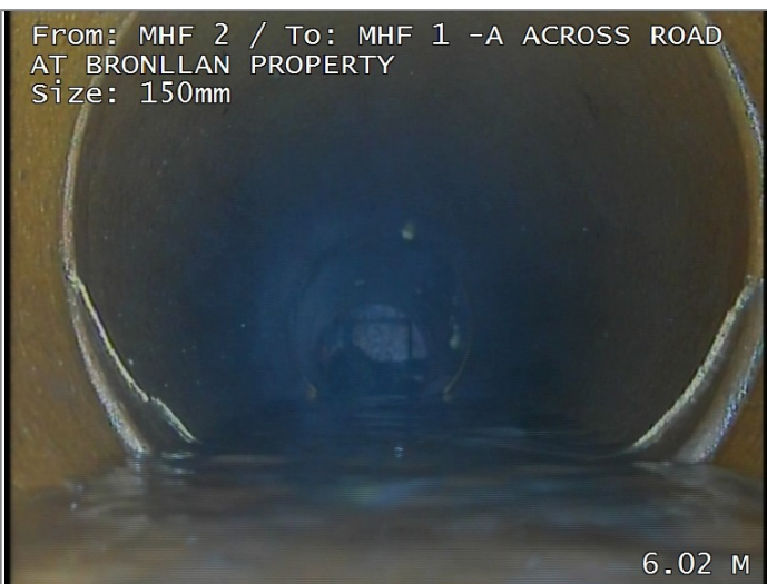
Crack circumferential from 3 to 9 o'clock
