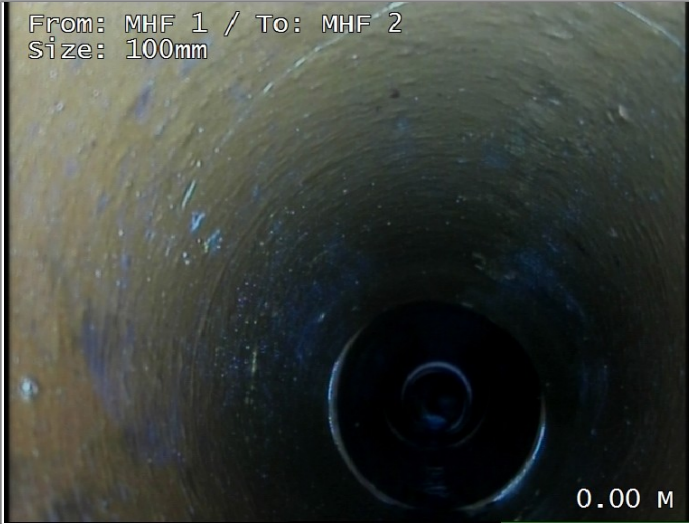
Crack circumferential from 12 to 12 o'clock
