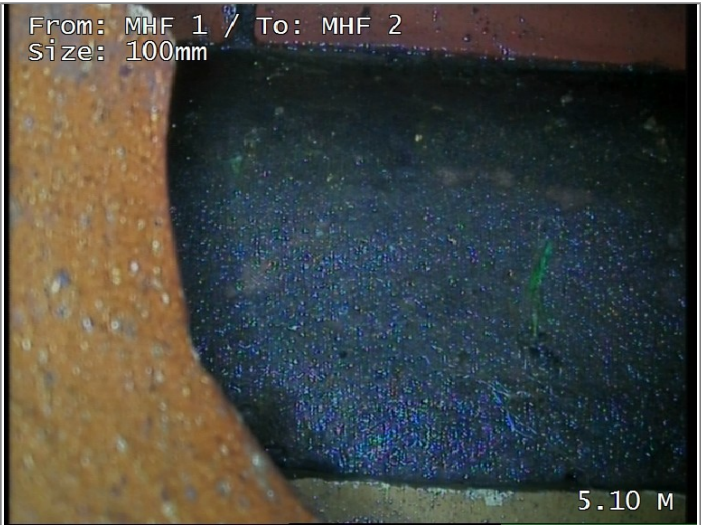
Finish node type, manhole, reference MHF 2
