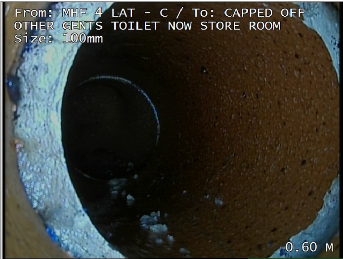
Crack circumferential from 10 to 2 o'clock
