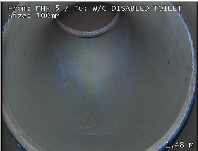
Line of drain/sewer deviates up
