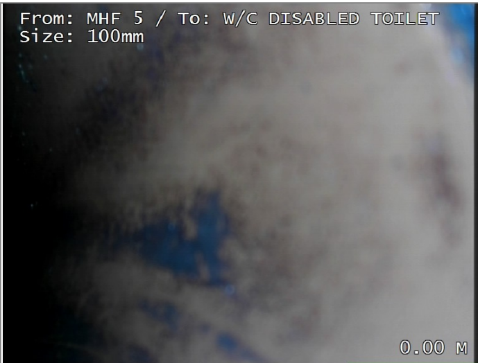
Line of drain/sewer deviates left
