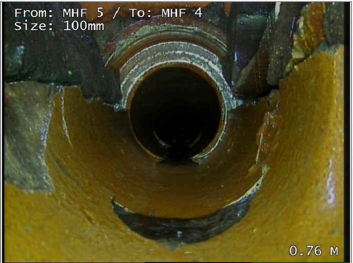
HOLE AND CRACK IN MAIN CHANNEL
