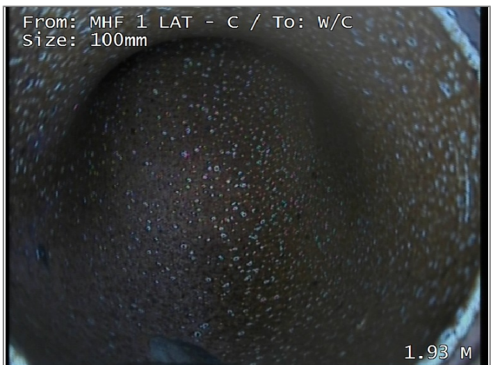
Line of drain/sewer deviates up
