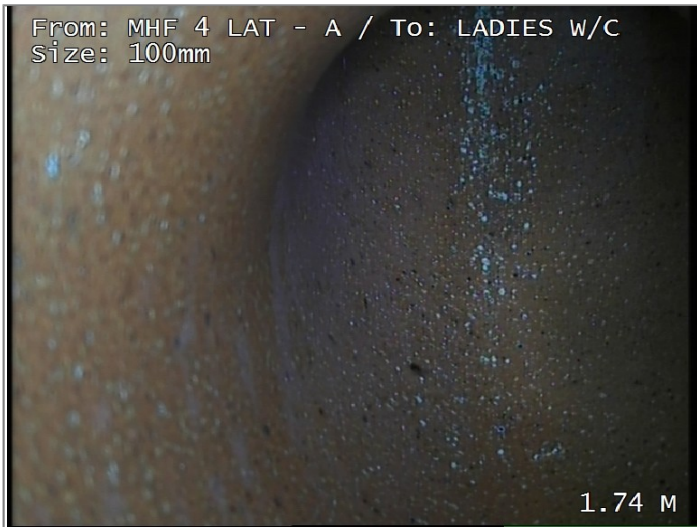
Line of drain/sewer deviates up
