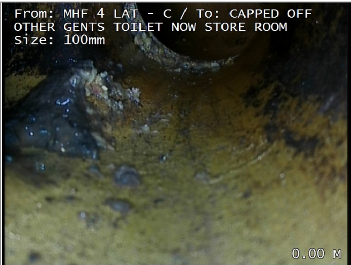
Junction at 9 o'clock, diameter 100mm - Remark: SVP JUNCTION
