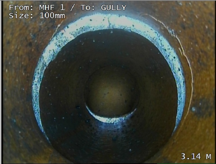
Crack circumferential from 12 to 12 o'clock
