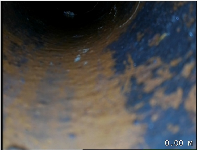
Start node type, manhole, reference MHF 2 LAT - B
