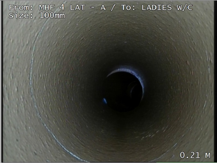
Crack circumferential from 12 to 12 o'clock
