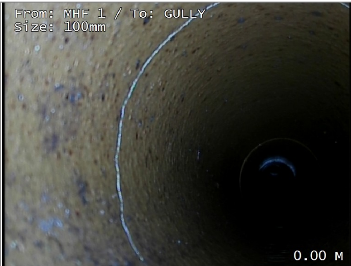
Crack circumferential from 12 to 12 o'clock
