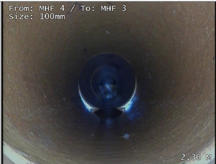
Crack circumferential from 8 to 12 o'clock
