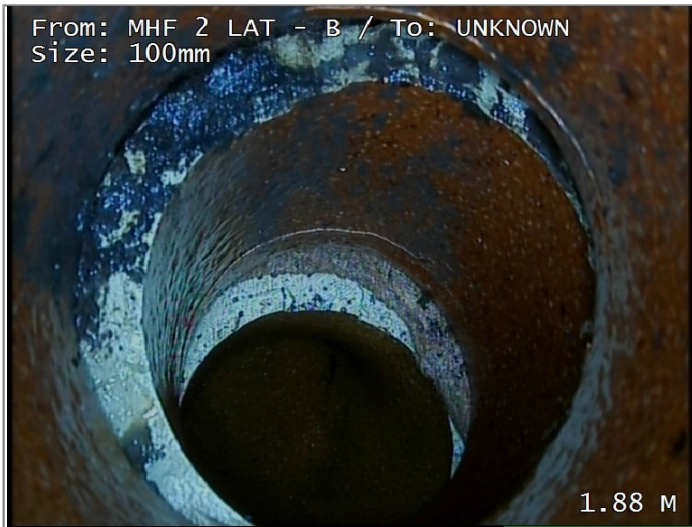
Joint displaced large
