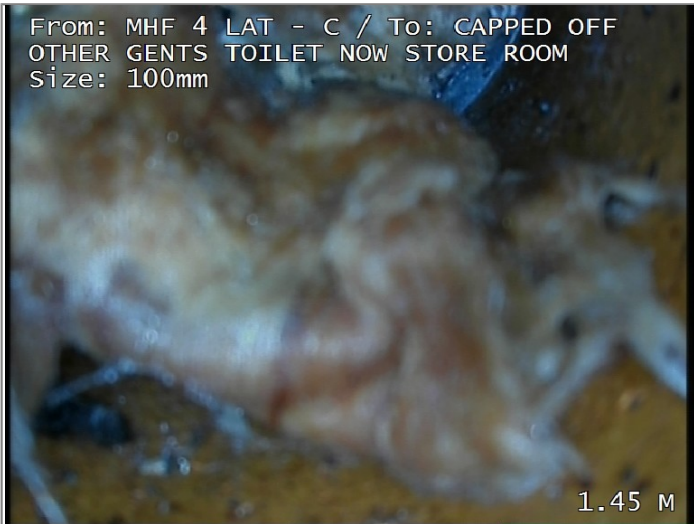
Finish node type, major connection without manhole, reference CAPPED OFF OTHER GENTS TOILET NOW STORE ROOM
