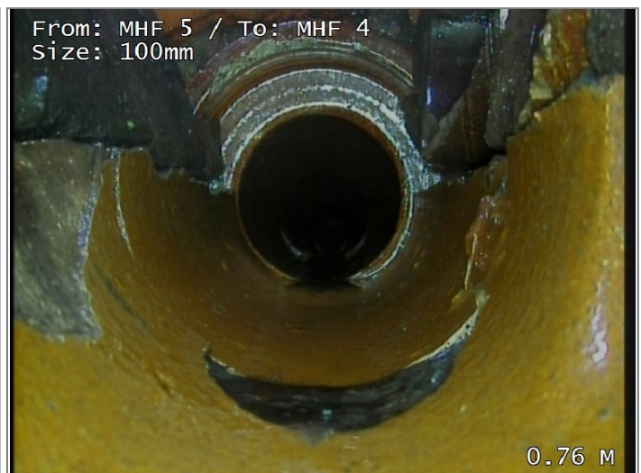
Crack circumferential from 2 to 10 o'clock
