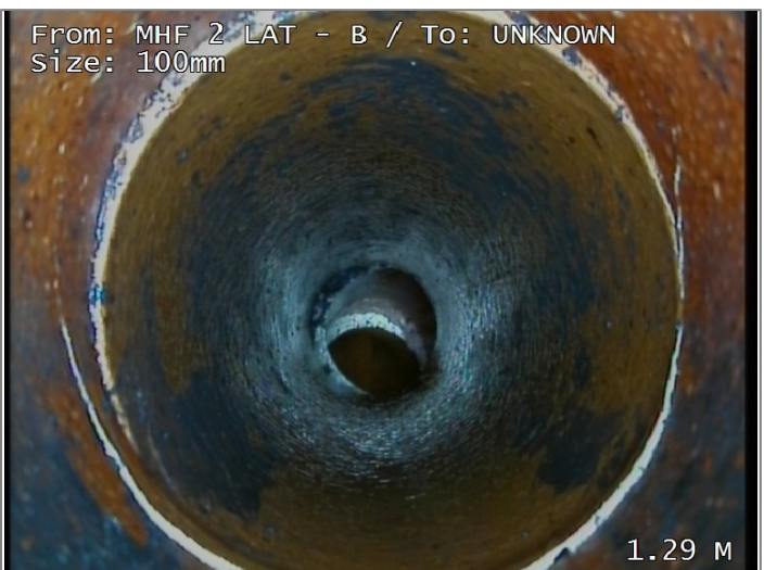
Crack circumferential from 2 to 10 o'clock
