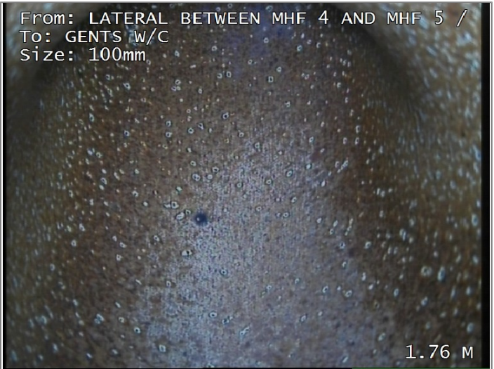
Line of drain/sewer deviates up
