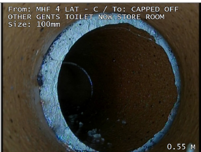
Joint displaced medium
