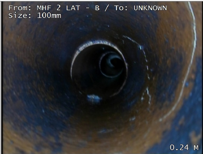
Cracks multiple from 12 to 12 o'clock
