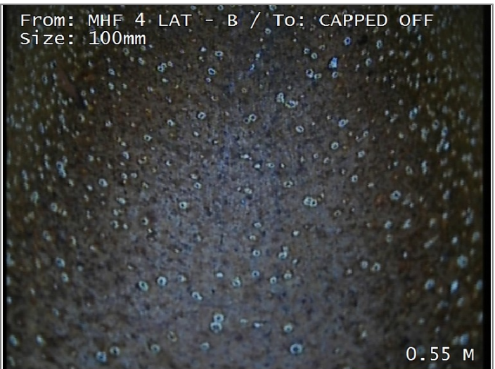
Line of drain/sewer deviates up
