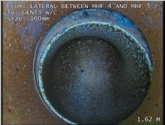
Joint displaced medium
