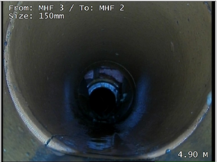
Cracks multiple from 12 to 12 o'clock
