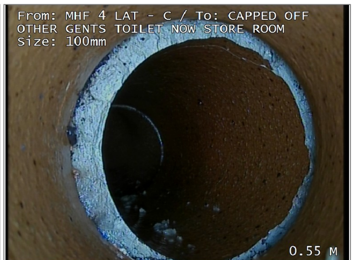
Line of drain/sewer deviates left
