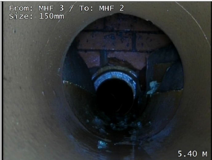
Crack circumferential from 12 to 12 o'clock
