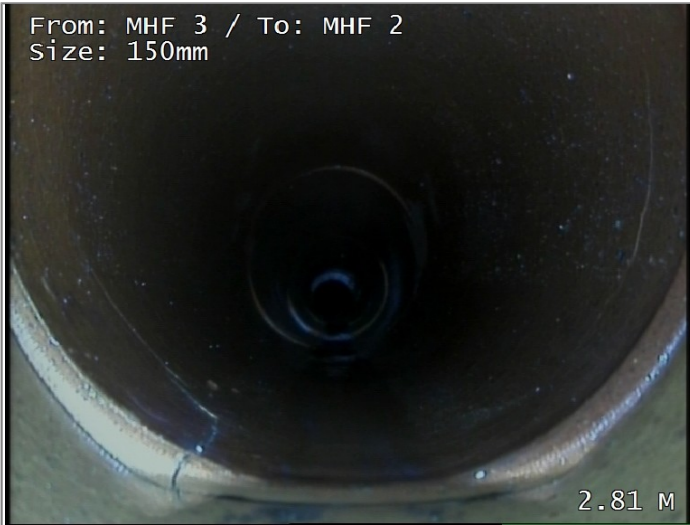
Cracks multiple from 12 to 12 o'clock
