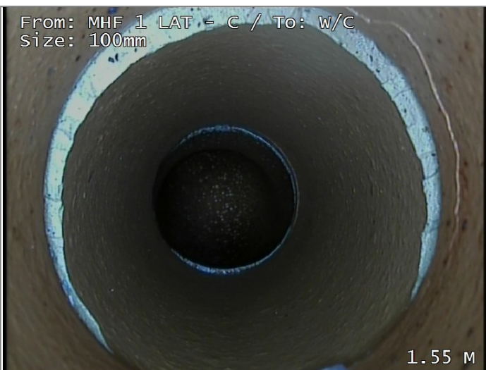
Crack circumferential from 12 to 12 o'clock
