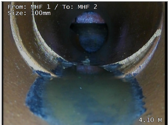
Crack circumferential from 2 to 10 o'clock
