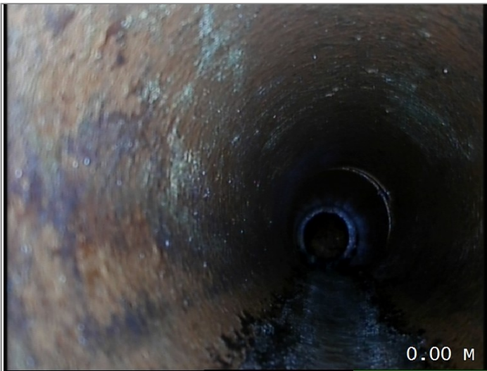
Start node type, manhole, reference MHF 1 LAT - A
