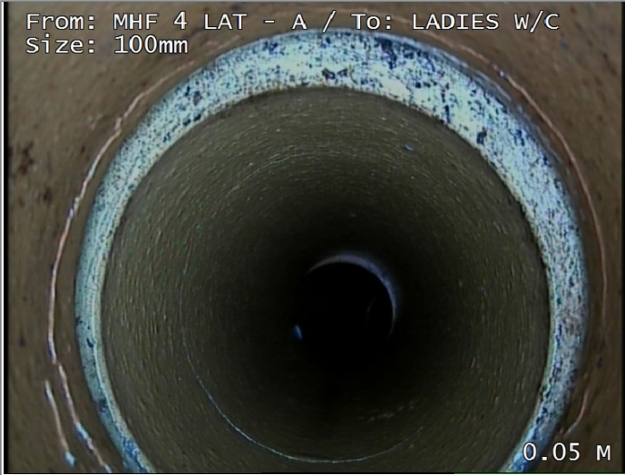
Crack circumferential from 12 to 12 o'clock
