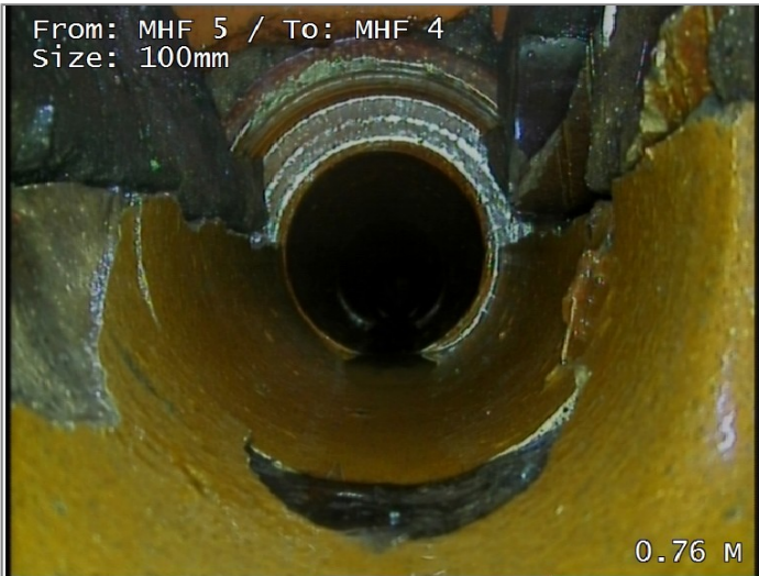
Finish node type, manhole, reference MHF 4
