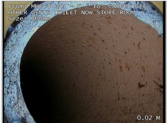
Line of drain/sewer deviates left
