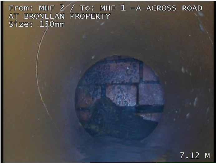
Crack circumferential from 12 to 12 o'clock
