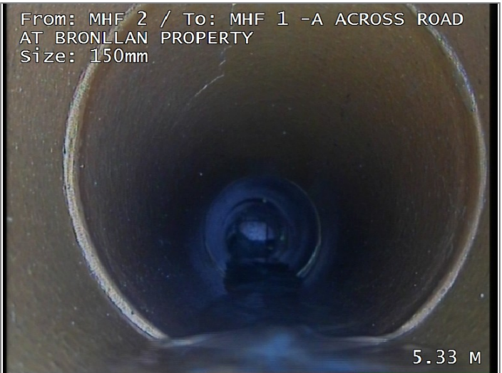
Crack longitudinal at 12 o'clock
